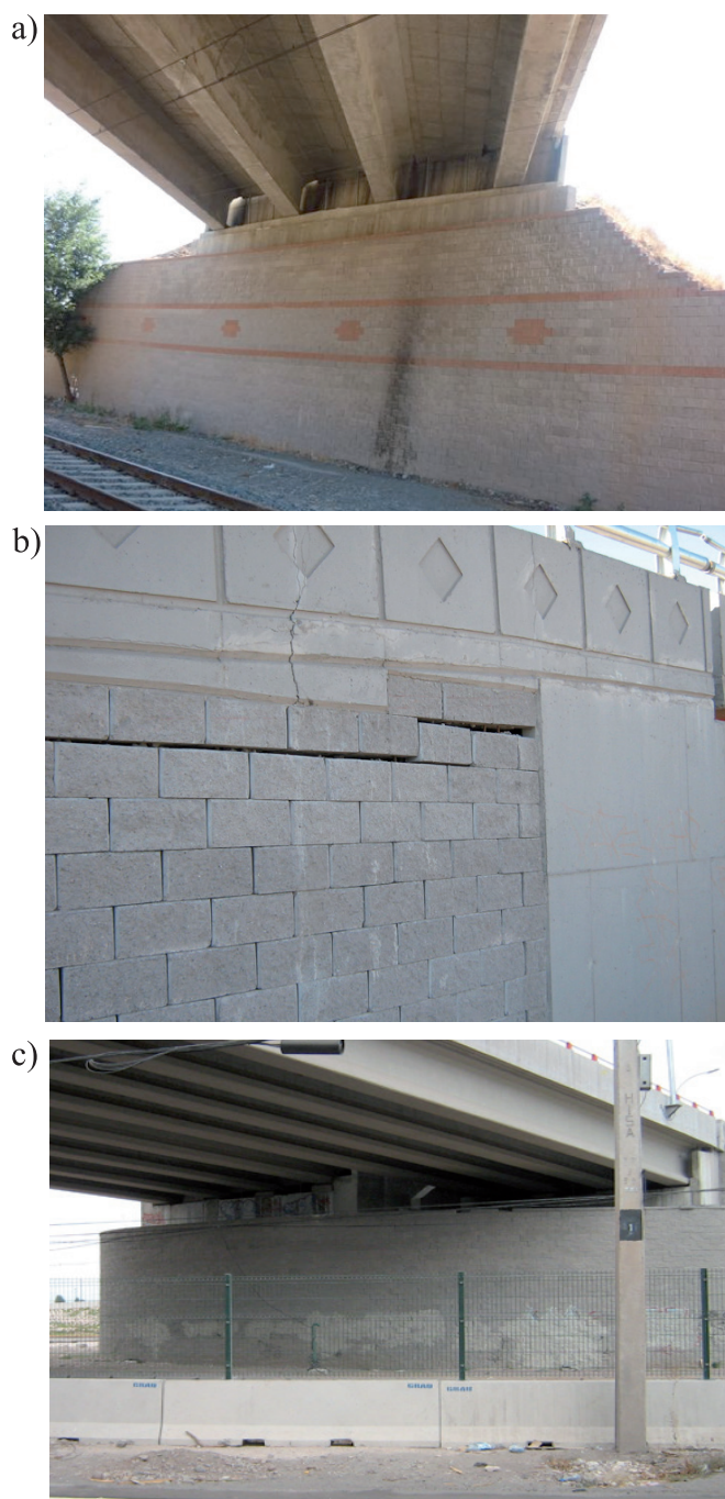
Figure 1: Pictures of geogrid reinforced soil walls after the 27F earthquake. a) No visible movement in bridge abutment wall in San Francisco de Mostazal, b) block vertical movement and fissures in Bonilla roundabout overpass and c) curved abutment in the overpass of Ruta 78 junction in Pajaritos Avenue without noticeable movement
