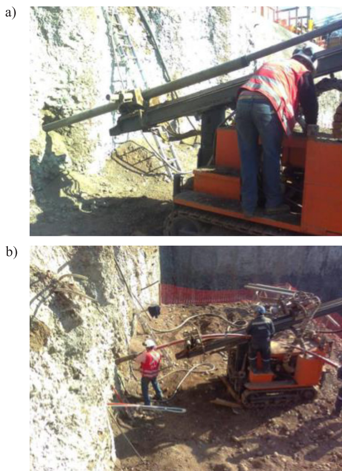
Figure 6: Installation of Energy Anchors: a) ground drilling, and b) cable and HDPE pipes are inserted.
