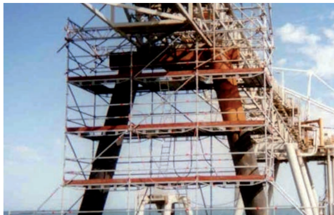
Figure 1: Bridge piles under corrosion control and maintenance.
